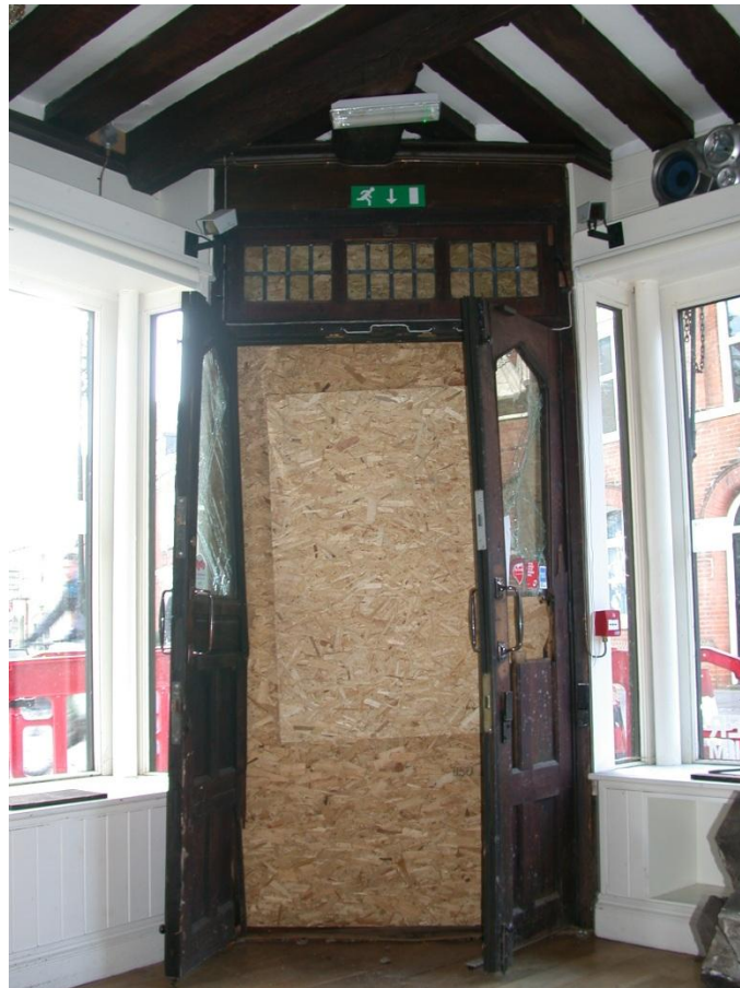
The damaged front doors. Remarkably the door frame itself has survived intact as have the two adjacent cast iron struts.
