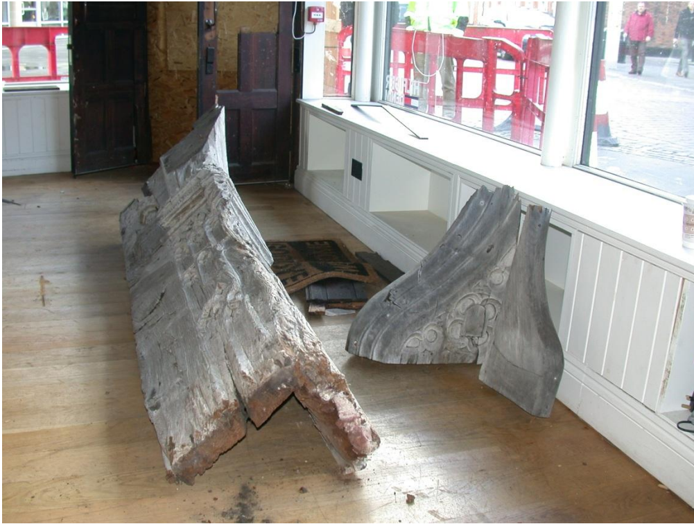
Inside the property a few days after the crash. The “L” section of the corner post can clearly be seen; to the right is a bracket and the 1902 (?) repaired section from the top of the post. In the background the damaged front doors still in-situ.
